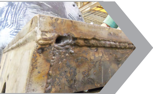
POOR WELDS AND CONSTRUCTION OF THE EXISTING FAN CAUSED EXCESS VIBRATION
