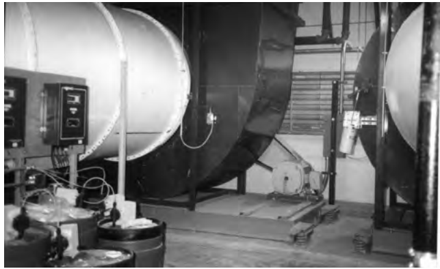
Figure 5. Fan mounted on an inertia base
