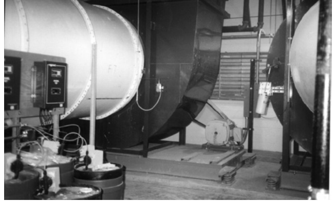
Figure 5. Fan mounted on an inertia base
